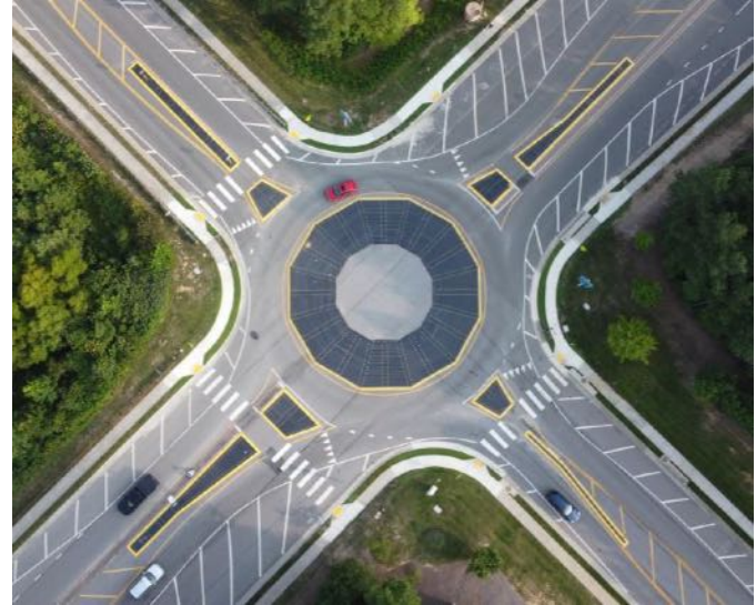
Actual installation of the Vortex modular system by maintenance crew or sub-constructor
